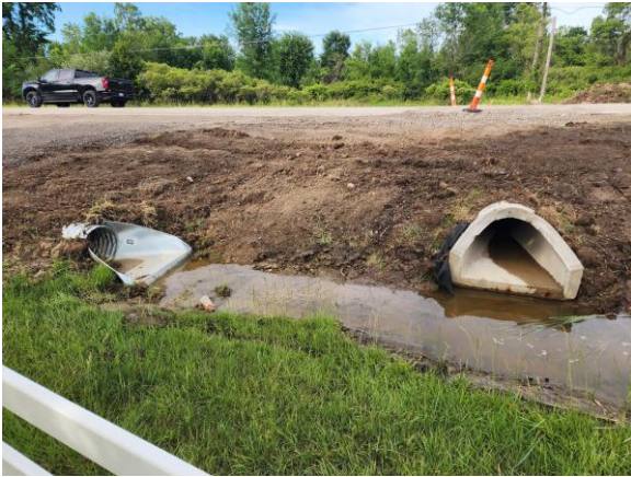
Jun 2026 — cross culvert discharging east onto private land.
