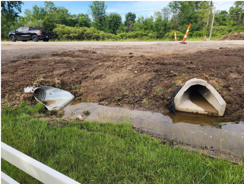
Exhibit D1 — Jun 15, 2026: the cross-road culvert outlet on the east side (old flattened pipe at left, new concrete box at right) discharging water onto private land behind the white fence.
