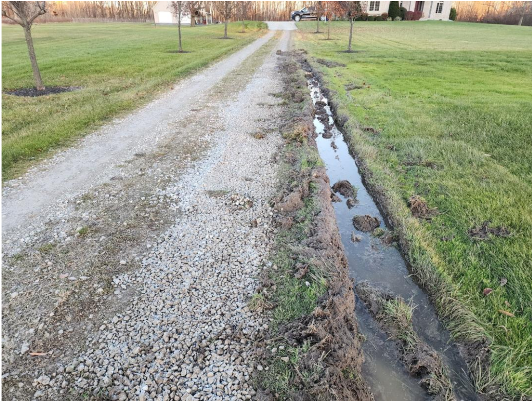
Exhibit A2 — Nov 24, 2024: fast-moving water has cut a deep eroded channel along the edge of the limestone driveway.
