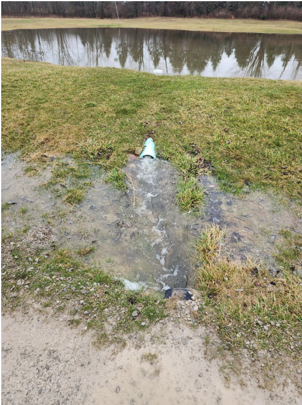
Exhibit A1 — Mar 31, 2023: a drainage outlet discharging a concentrated flow onto the property; standing water beyond. The problem long predates the 2026 road work.
