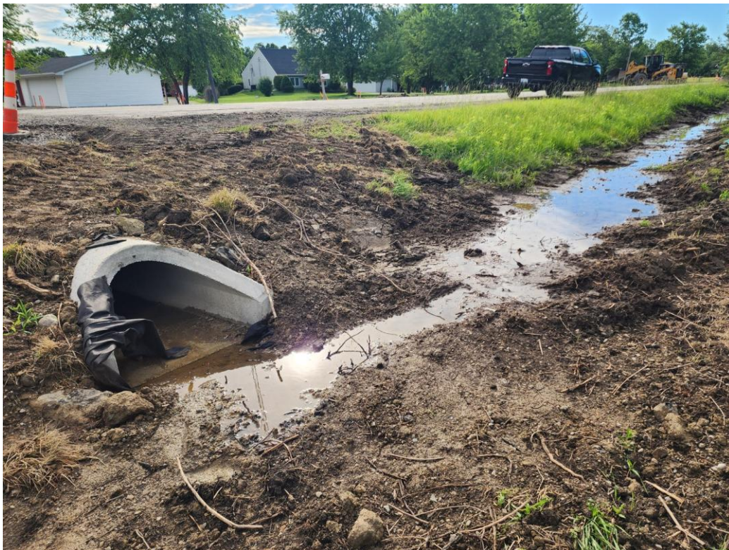
Exhibit D2 — Jun 15, 2026: that discharge running into a shallow, freshly graded ditch on private property — not a road ditch.
